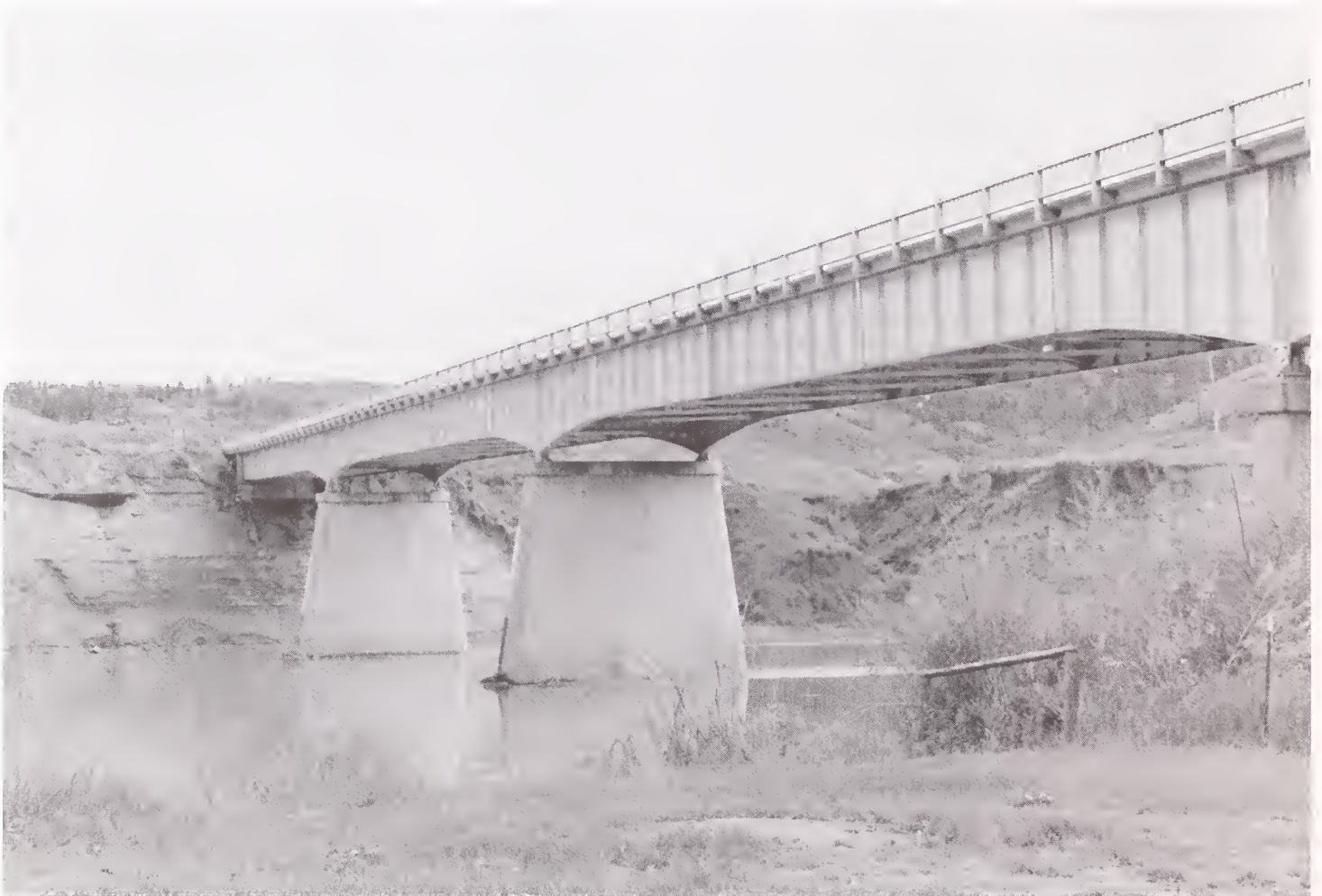
The Fred Robinson Bridge is a steel girder and floor beam bridge built between 1955 and 1959.
